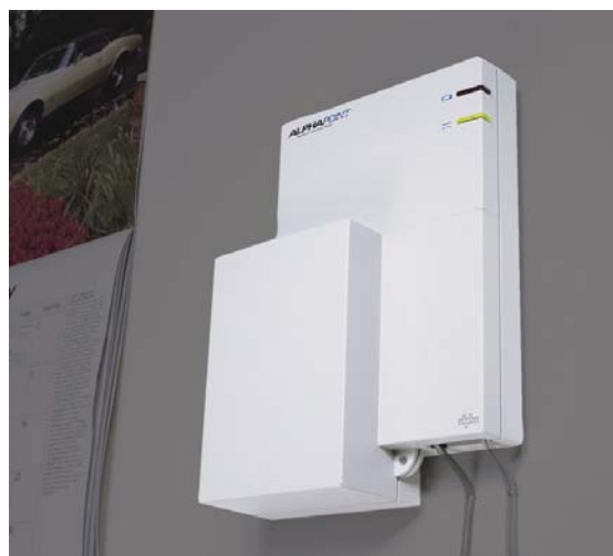
Early generation indoor premise ONT power supply typically installed indoors
