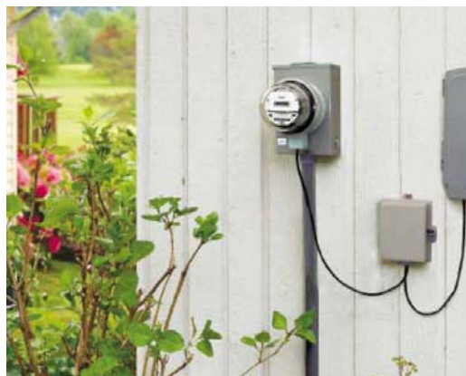
AC to DC power converter installed in a socketed meter collar and an 18 Watt battery module supporting the ONT at the home
